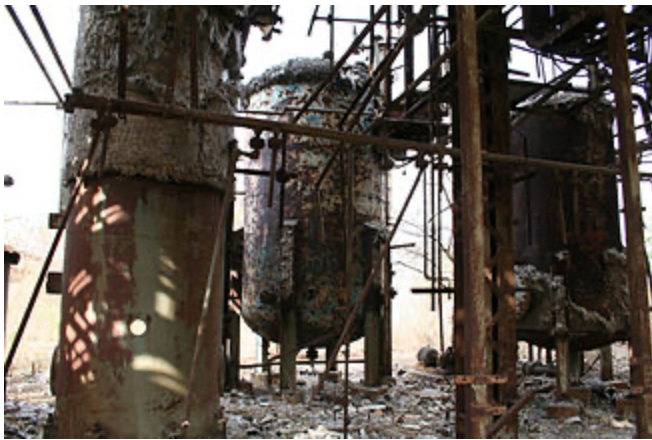
Deteriorating section of the MIC plant, decades after the gas leak.
